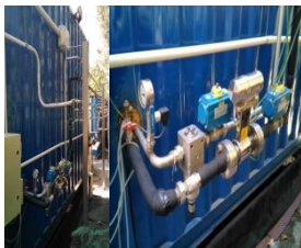
Figure 83: External air and water ducts
