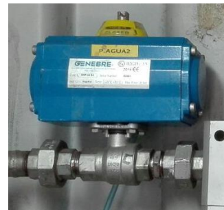
Figure 80: Water pressure valve
