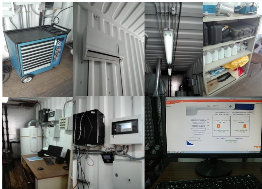
Figure 55: Equipment of the Control Room
