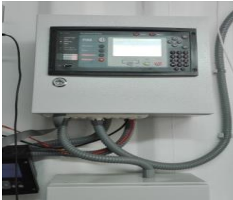
Figure 65: Remote smoke alarm control panel
