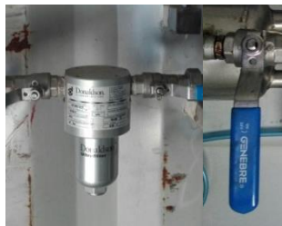
Figure 77: Air filter for the air and water pressure system and ball valves
