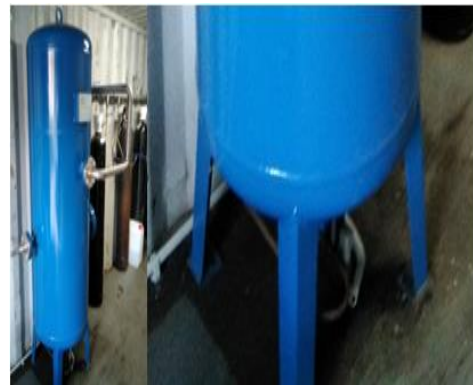
Figure 70: Pressurized air tank and drainage sensor
