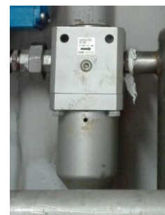
Figure 81: Manual water pressure regulation valve
