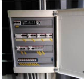
Figure 76: Electrical protectors box of the Machinery Container
