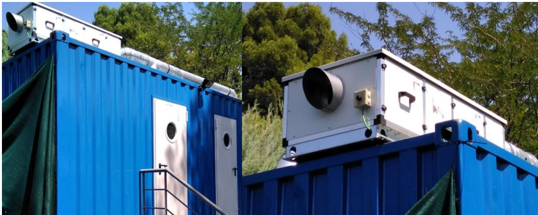
Figure 45: Ventilation system and filters
