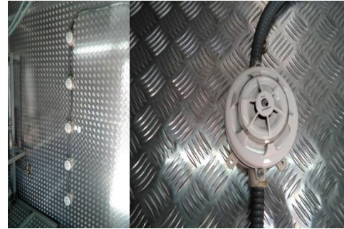
Figure 48: Smoke particle detector system
