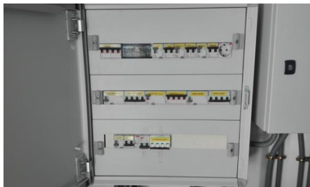
Figure 61: Electrical protectors box of the Test and Control Container
