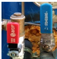
Figure 85: External circuit manual ball valves
