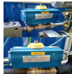
Figure 87: Air and water pneumatic valves
