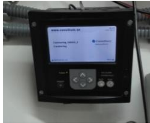
Figure 66: Remote control panel for fire detectors
