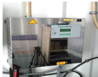
Figure 64: Humidifier/dehumidifier control panel
