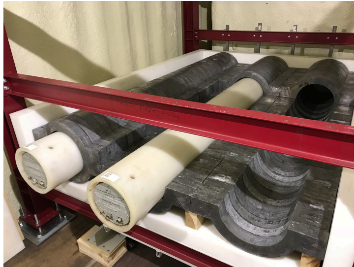
Figure 5.16: NEMO 3NM64 section during construction. 240 lead pieces weighing around 21.4 kg are used, and the total weight is almost 6 t.
