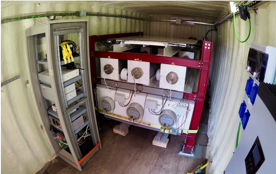
Figure 5.18: Complete ORCA arrangement inside the container, after installation at the base.
