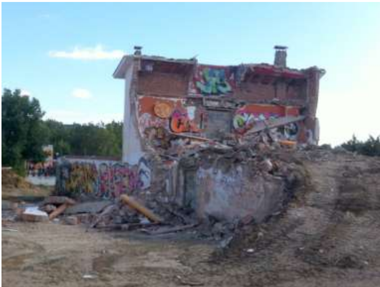
Fig. 51. An abandoned discotheque building next to the school playground, which became a hide out for young people and was recently pulled down. (Photograph by author)
