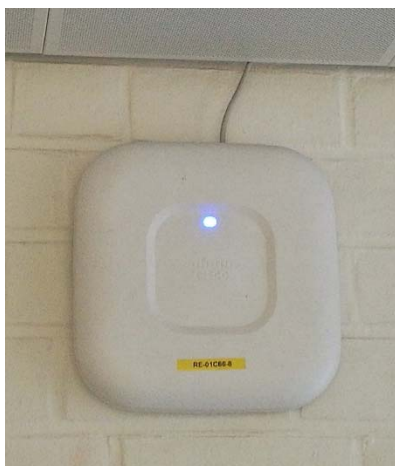
Figure 32 Wrong Placement of an Omnidirectional Antenna
