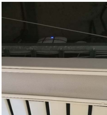
Figure 33 Wrong Placement of an Access Point
