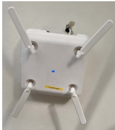
Figure 34 Wrong Placement of Antenna on a Directional Antenna
