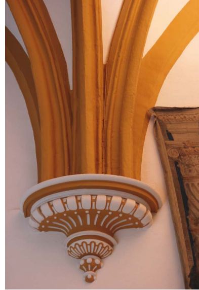
Fig. 7. Detail of the vaults of the upper floor of the 'Gothic palace', Seville Alcázar, late thirteenth century? (Photo: Tom Nickson).
