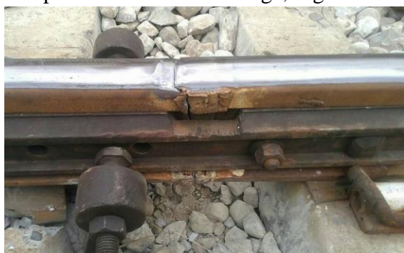
Fig. 1-1 An example of track breakage
