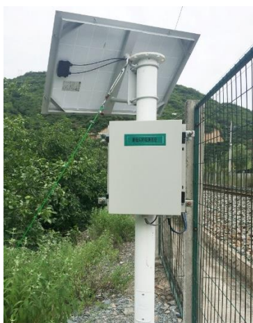
Fig. 4-4 Power supply unit for each node of track breakage detection system
