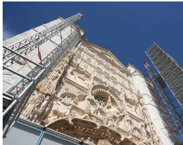
Fig. 14. The façade without the scaffolding and with the lift platform that permitted to document the final result of the restoration works
